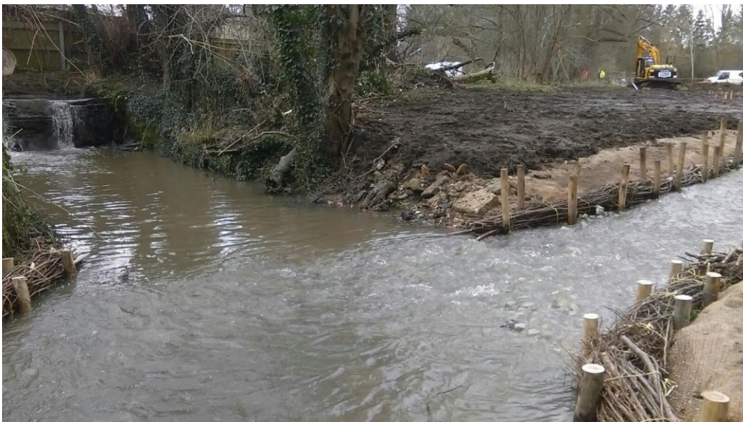
Photo 2 - A newly constructed nature like bypass channel around an impassable weir (visible to the left) on the River Darent, Kent.
