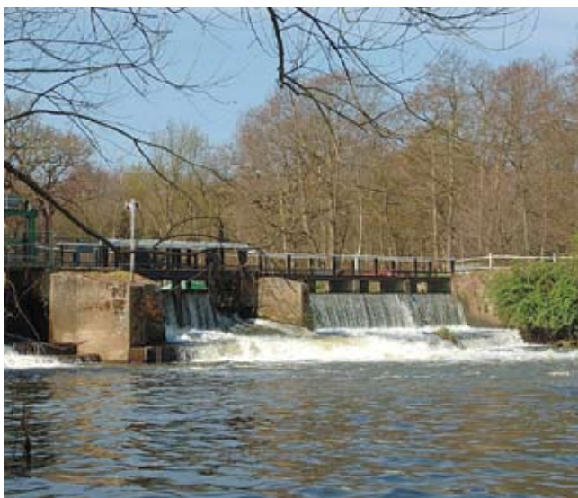
Walsham Weir, River Wey-Ripley
