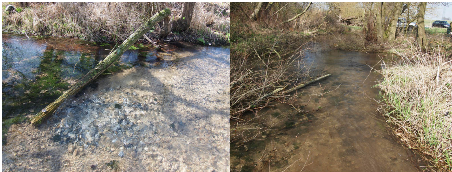
Completed Large and Coarse Woody Debris installation on the River Whitewater, March 2012. © John Sutton, 2012
