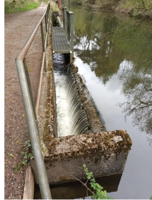
The Gelvert overflow
